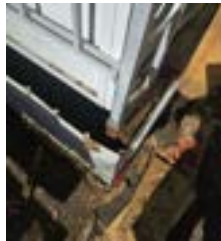
Rotted deck to be replaced
