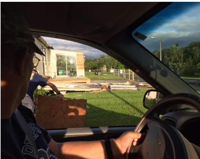
The first look at WG Lions Club House in Orange Trailer Park. The entrance way and carport were destroyed making the rest of the building unusable at this time. WG Lions are without their home!
