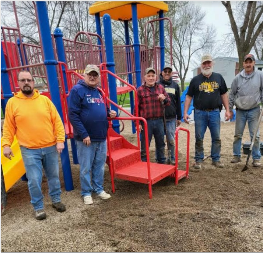
Lucan Lions participated in helping with cement work at the playground in the park. Pictured: Mike Schieber, Lion Greg Janachovsky, Lion Terry Ourada, Chris Kramer, Lion Dave Ourada, Lions Dennis Plaetz.
