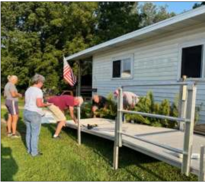
Lakefield Lions installed a ramp for a local recedent to use during recovery. They have two ramps to utilize in the area.
