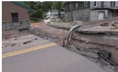
WNEP Television Station: Trout Run roads completely gone down river
